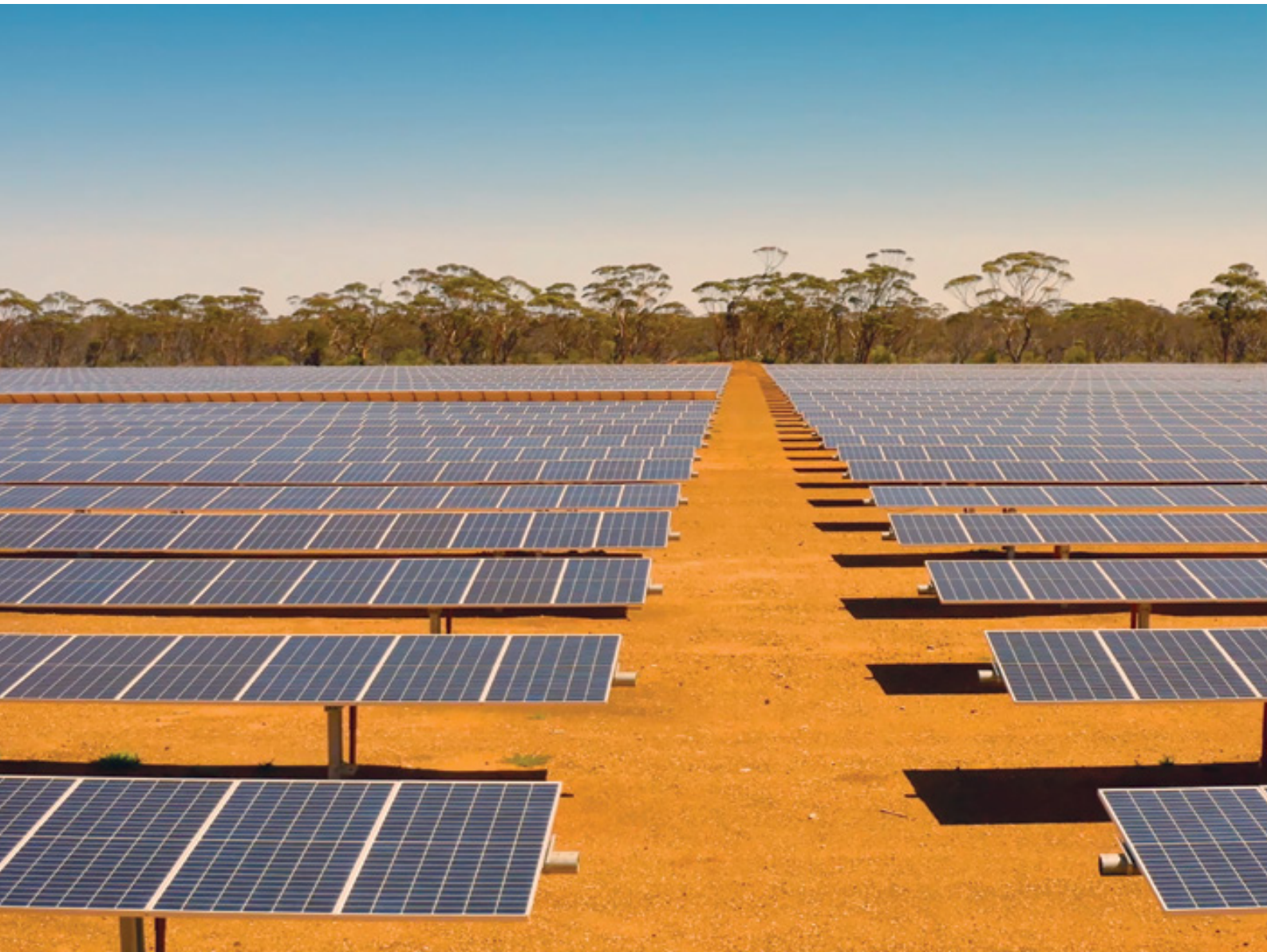
Nova Operation 5.5MW solar farm
