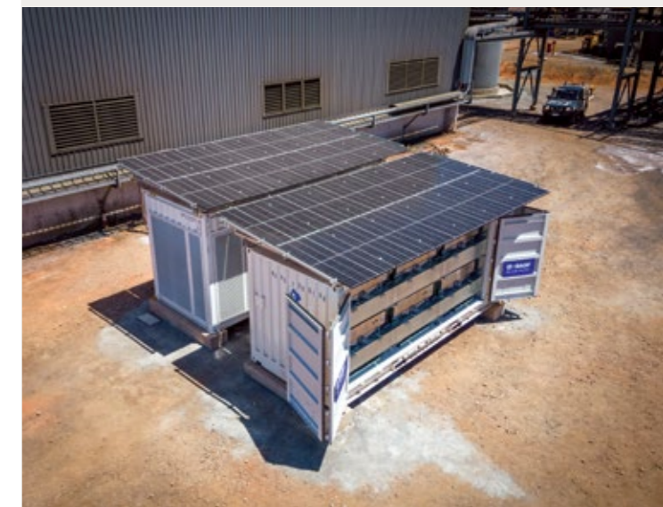
NaS Battery at our Nova Operation
