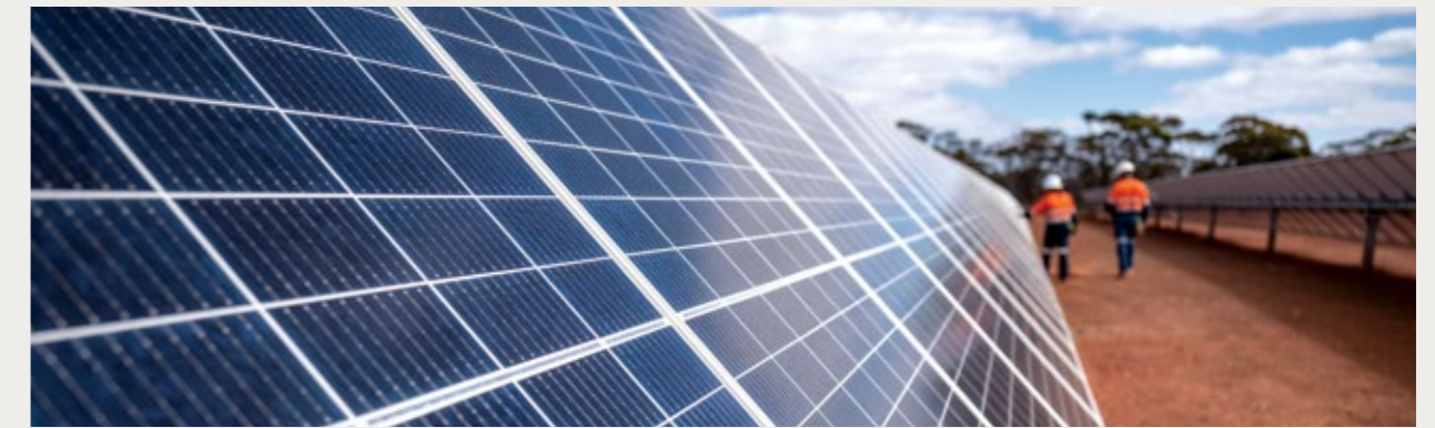
Nova Solar Farm
